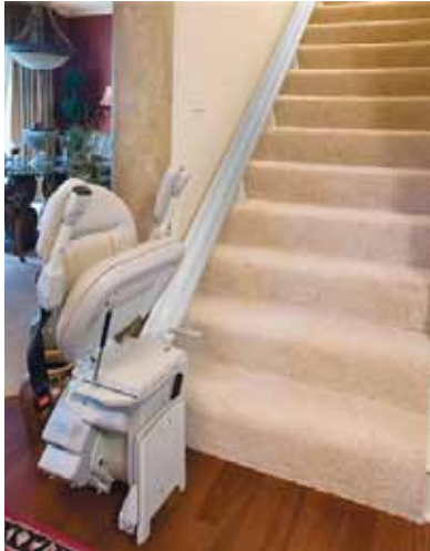
Indoor electric stairlift positioned at the bottom of the staircase.
